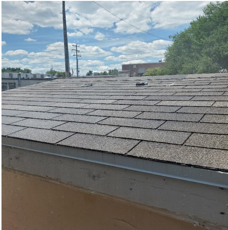
Photo No. 3 35 MPH Top Side
