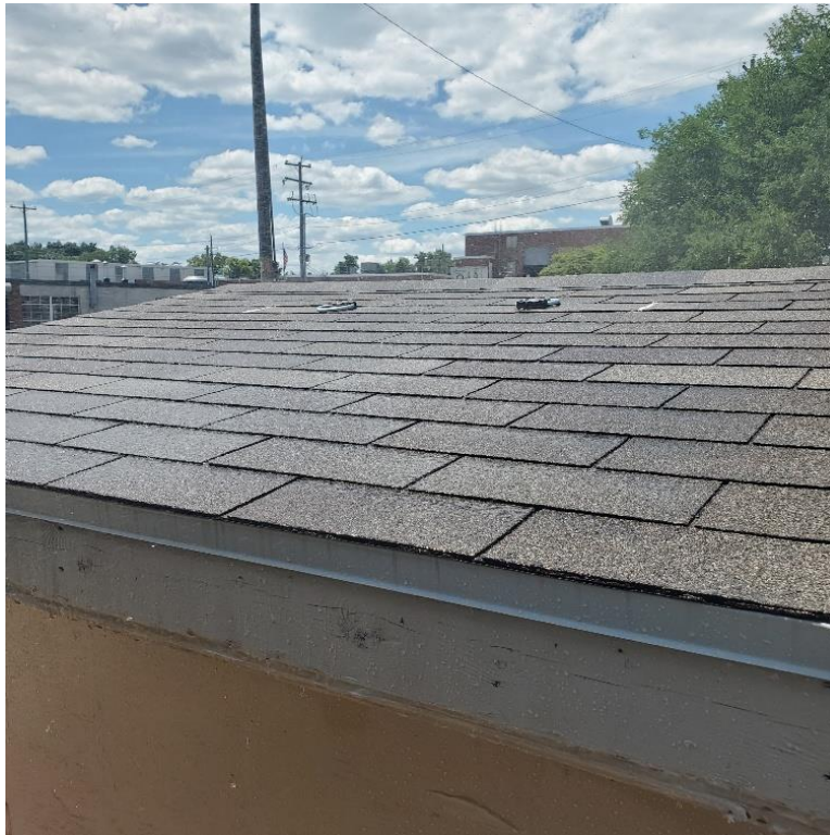
Photo No. 7 90 MPH Top side
