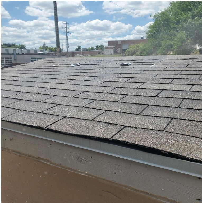
Photo No. 9 110 MPH Top Side
