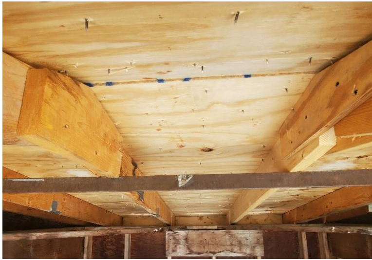
Photo No. 12 Post Test Underside
