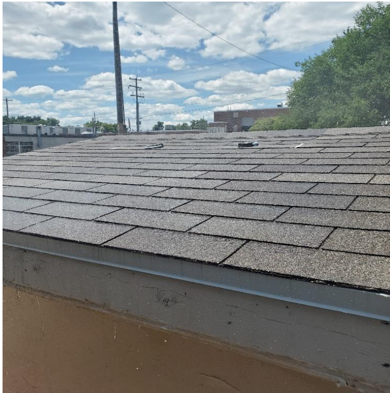
Photo No. 5 70 MPH Top Side
